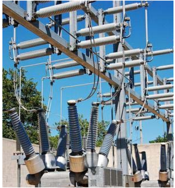
\text{SF}_6 is used in high voltage power system (Photo credit unknown)
